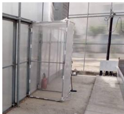
Picture 4. Entrance in the solar drying unit with insect protection
