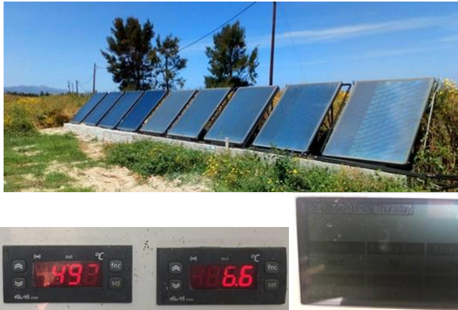
Picture 2. The heating pump and 4 more new solar panels
