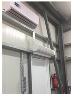
Picture 3. Two air curtains have been added in the doors of the pretreatment unit
