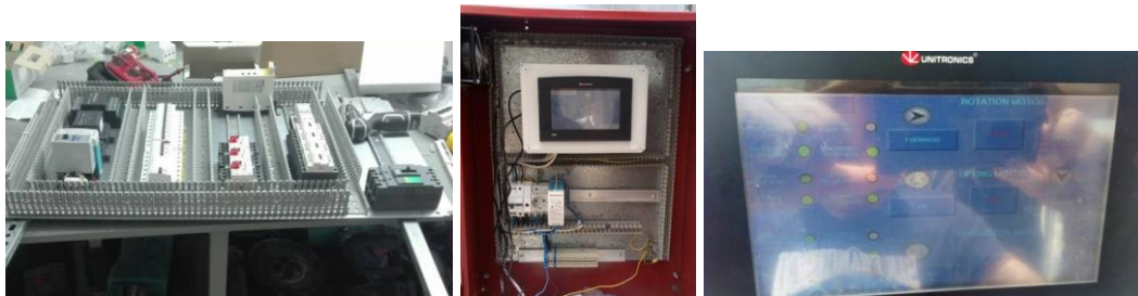
Picture 4. Construction of the electrical panel and a PLC of the horizontal turner
