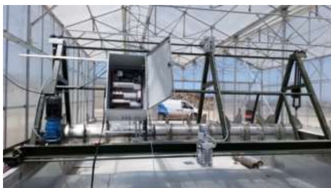
Picture 21. Placement of the electrical panel on the horizontal turner
