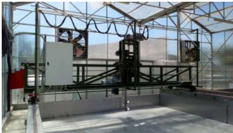
Picture 25. The installed vertical drying turning system on the drying hall
