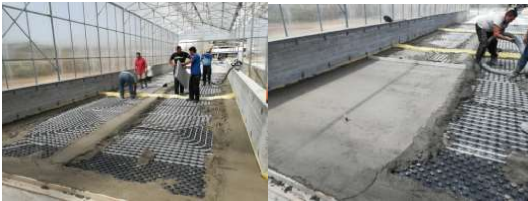
Picture 11. During the installation of the network of pipelines connected with water solar heater system
