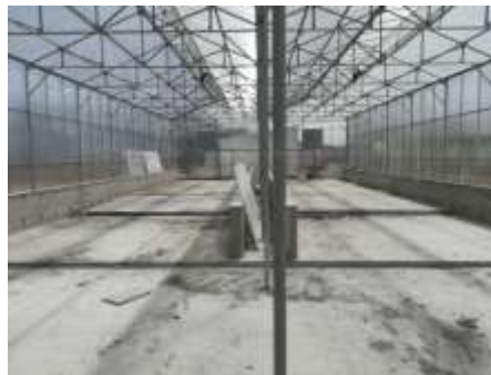
Picture 12. After covering with concrete the network of pipelines connected with water solar heater system
