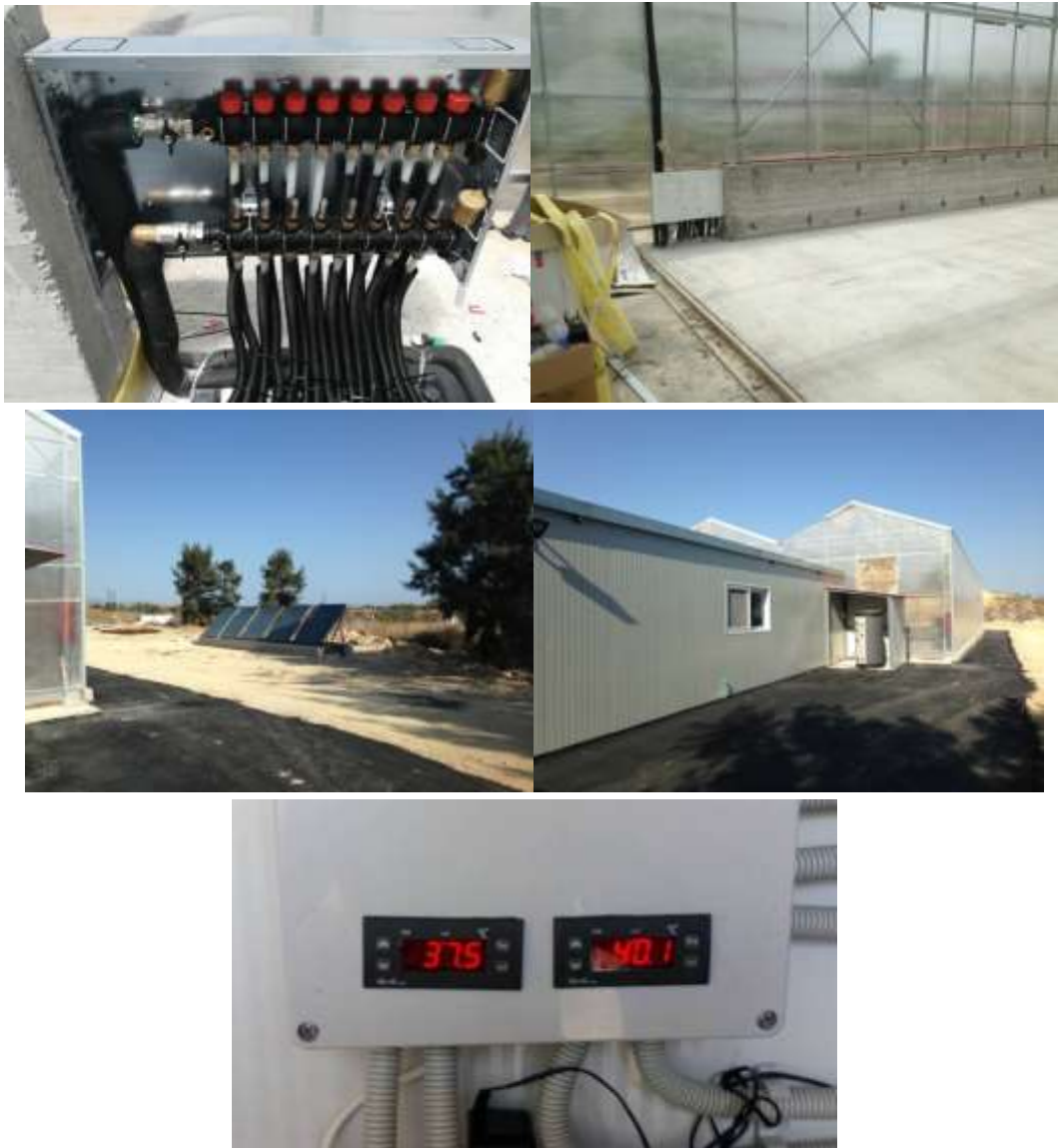
Picture 13. The heating system with the supply and return collectors, the boiler, the solar panels and the temperature display panel of the network of pipelines for the floor heating system
