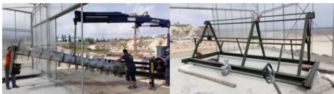
Picture 18. During transportation into the pilot unit
