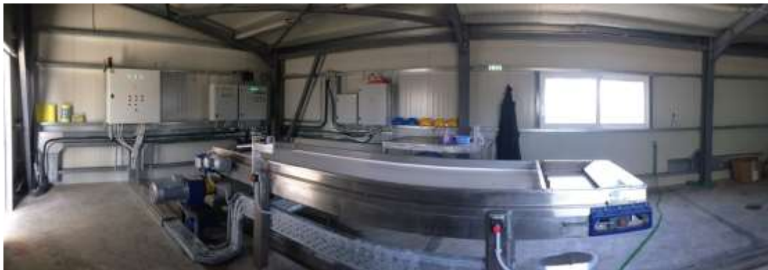
Picture 27. An overview from the interior of the pretreatment unit
