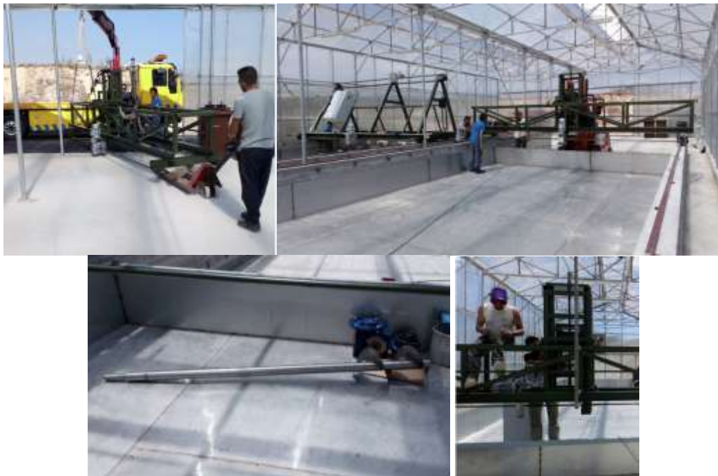
Picture 23. During transportation and installation of the vertical turner into the pilot unit
