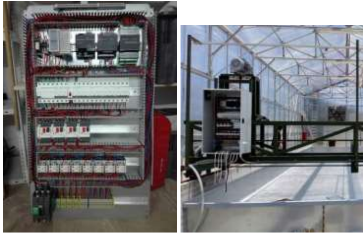
Picture 24. Construction of the electrical panel and a PLC of the horizontal turner
