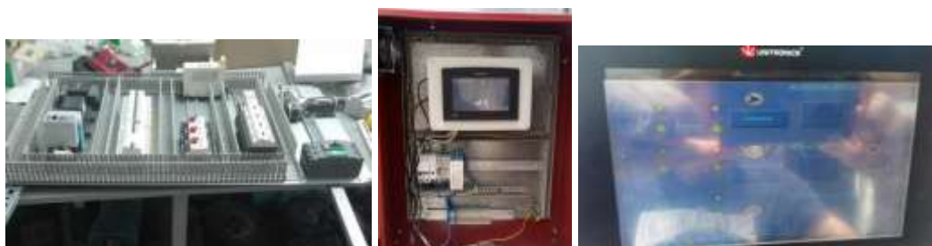
Picture 20. Construction of the electrical panel and a PLC of the horizontal turner
