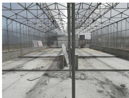
Picture 12. After covering with concrete the network of pipelines connected with water solar heater system
